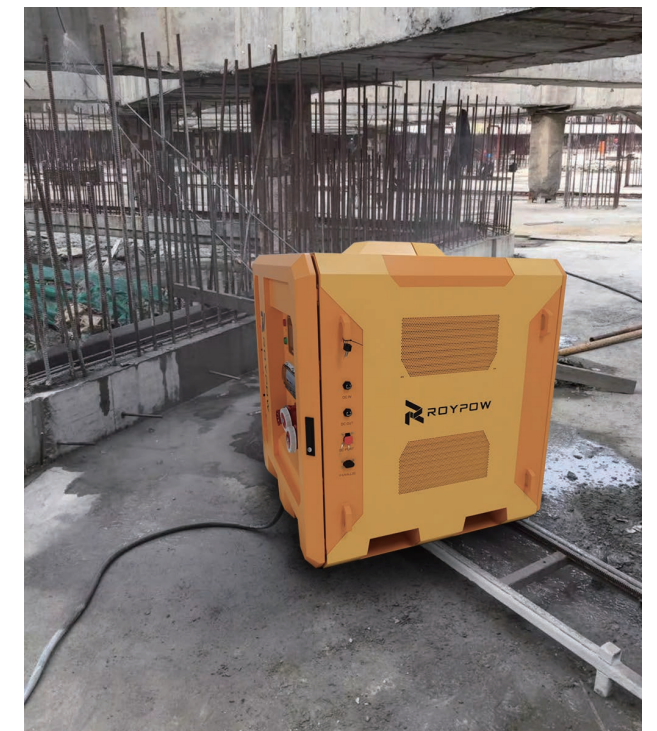
Construction Site Project Support Power Supply and Power Backup
