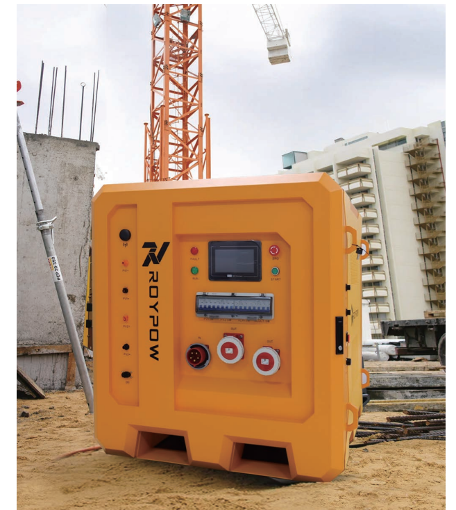
Construction Site Project Power Supply for Small Electrical Equipment
